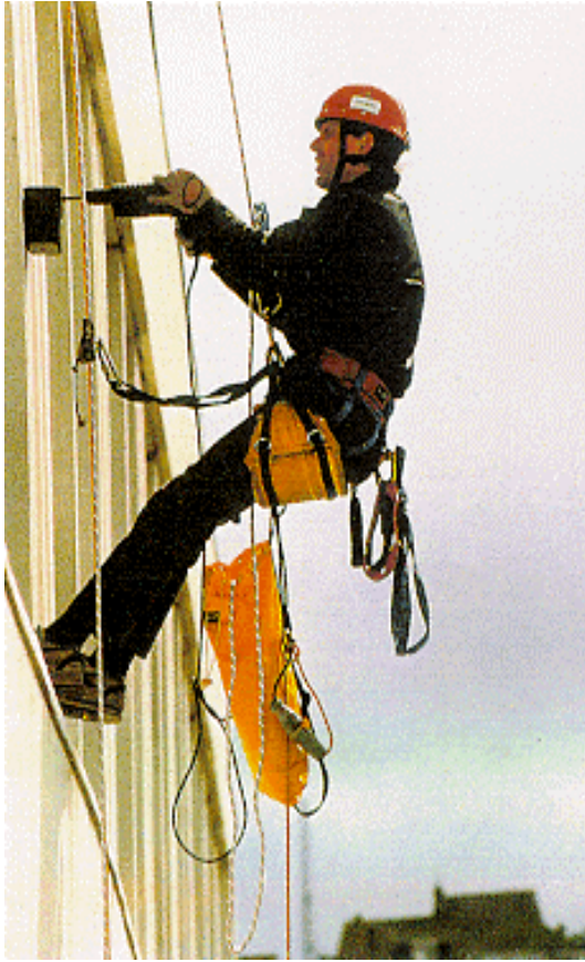
Inspection and material sampling of cladding by rope access (Photo: Messrs Sandberg)
