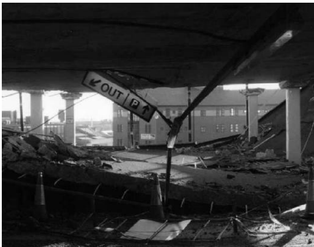
Partial collapse of the multi-storey car park in use at Pipers Row, Wolverhampton on 20 March 1997. (Photo: Wolverhampton Express and Star)
