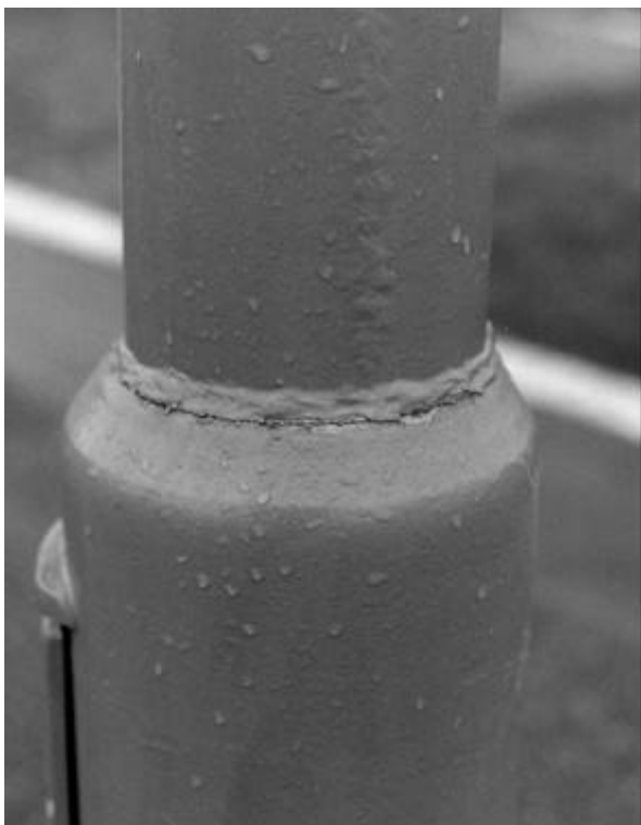
Fatigue fracture of a steel lighting column (Photo: Flint & Neill)
