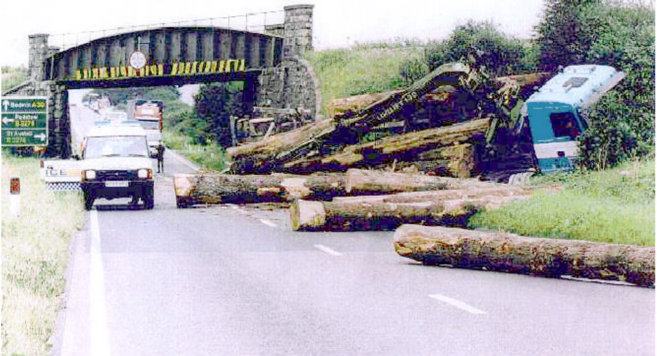
Structural Robustness: aftermath of a bridge strike by a road vehicle and its load on a railway underbridge (Photo: A3 Gross Moor Iron Bridge – Cornwall County Council)
