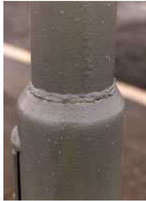
Fatigue fracture of a steel lighting column (Photo: Flint & Neill)
