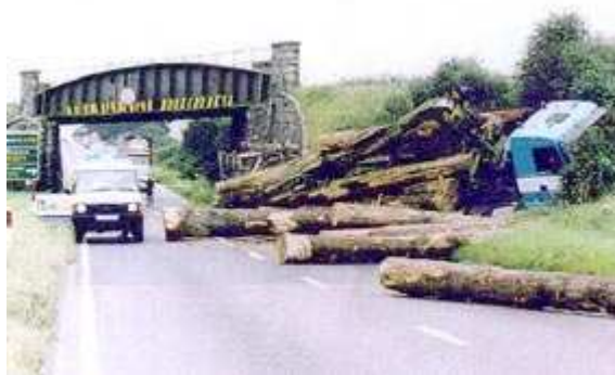
Structural Robustness: aftermath of a bridge strike by a road vehicle and its load on a railway underbridge (Photo: Cornwall County Council)
