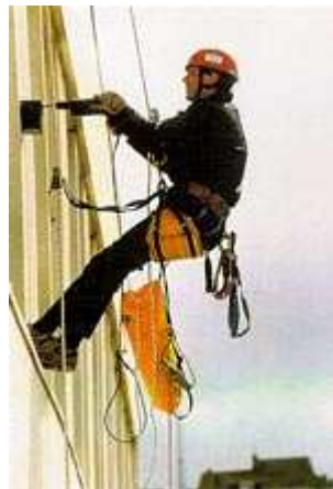
Inspection and material sampling of cladding by rope access (Photo: Messrs Sandberg)
