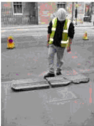
Fallen masonry from SCOTCROSS
