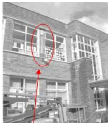
Column from which brickwork fell
