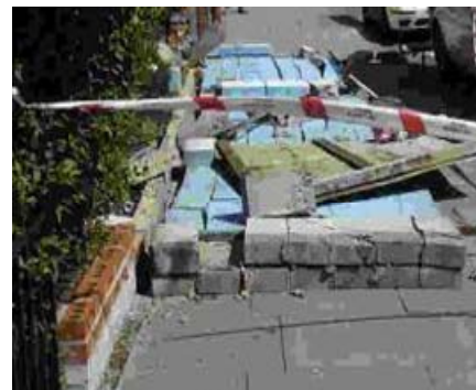
Collapse that caused death of a child (report 059 below)
