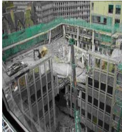
The collapsed floor
