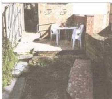
Collapse that caused serious injury (report 094 above)
