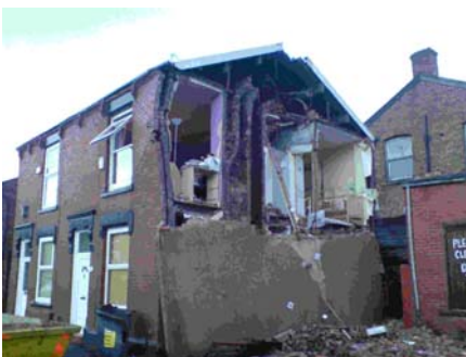
Collapse after failure to underpin
