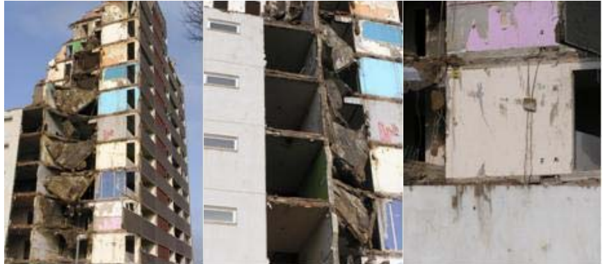
Photographs of the collapse of the second LPS block
