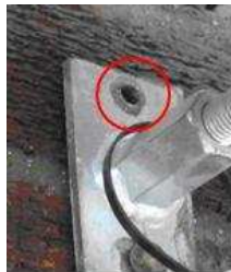
Image of bracket showing where fixing head has broken
