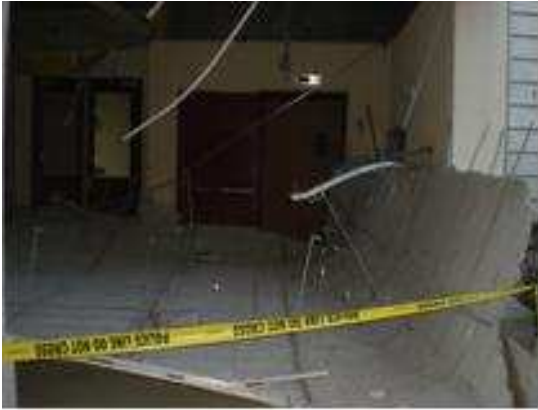
The collapsed ceiling
