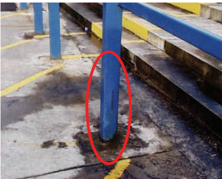
SCOSS Biennial report 2001: Split RHS due to freezing
