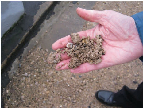
Loose aggregate on surface
