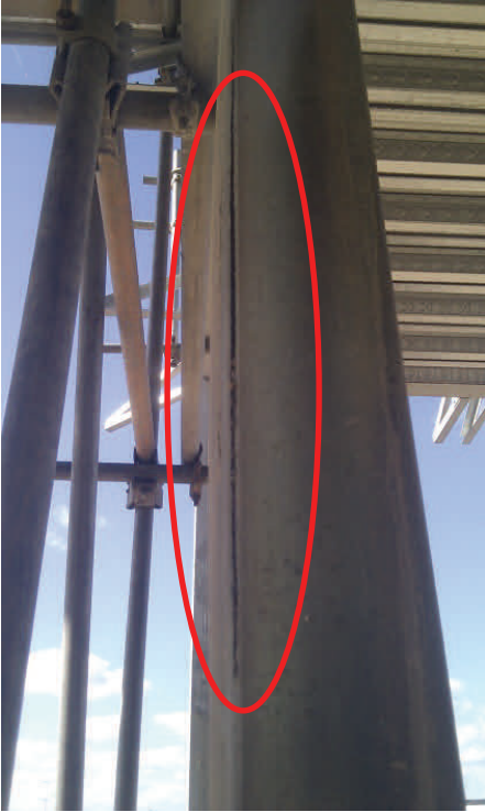
Report 253: Split RHS due to freezing
