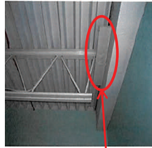
Typical connection: cleat bolted to beam and top flange of truss rests on cleat
