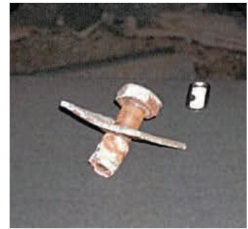
Failed bolt with part of shield still in place
