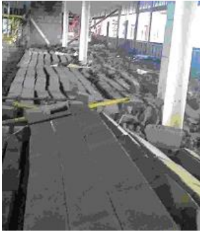
Internal wall that collapsed due to wind during construction
