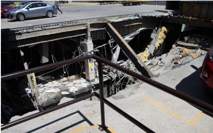
The collapsed roof structure
