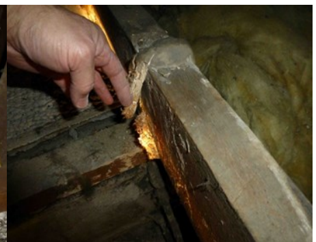
Another rotted connection
