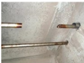
Fractured Tie Bar
