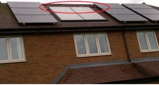
Outline shows area of damage
