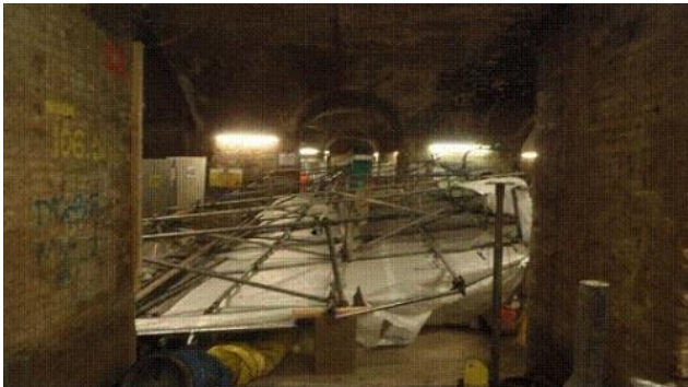
Underground scaffold blown over
