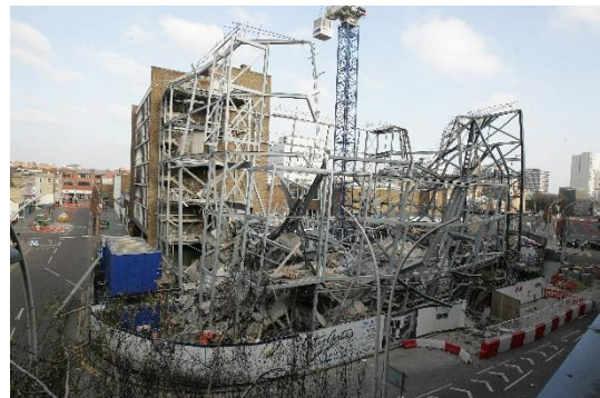
Figure 2: Collapsed structure Courtesy of the Ilford Recorder
