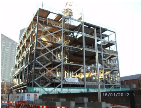
Figure 1: Fifteen days before collapse Courtesy of the Ilford Recorder
