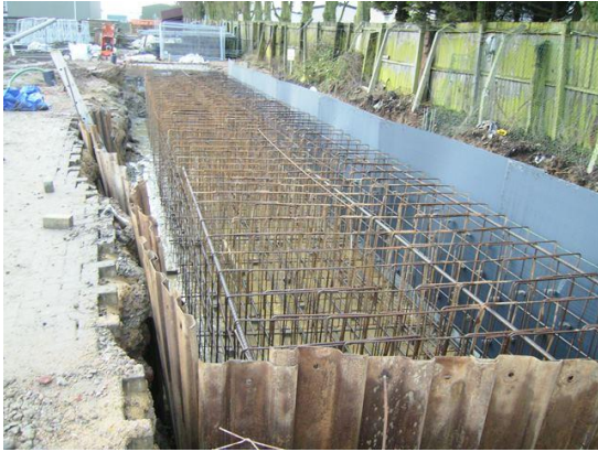
The rebar cage prior to collapse
