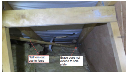
● Figure 3 Bracing deficiencies in the timber roof
