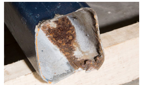
Figure 1 Failed support post
