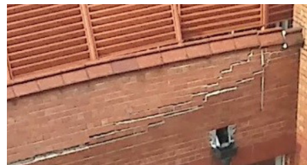
● Figure 2 Failure of masonry wall with fencing above
