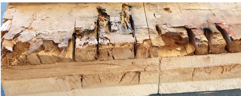
● Figure 1 Rotting of a CLT panel
