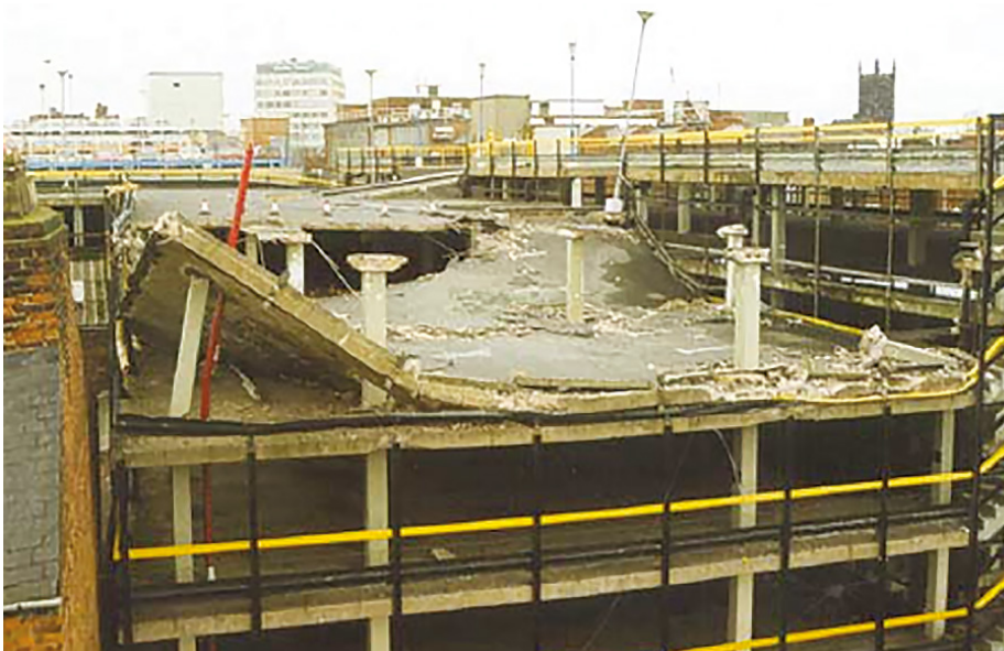
● Figure 2 Pipers Row car park collapse
