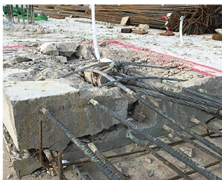
Figure 1 Post-tensioned slab failure
