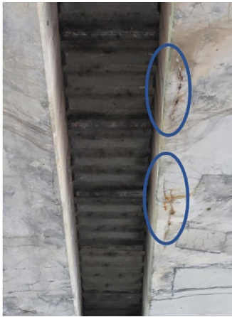
● Figure 1 Initial damage
