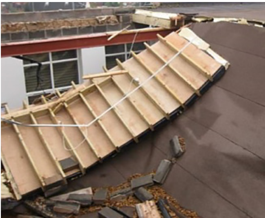
● Figure 5 Collapsed section of roof
