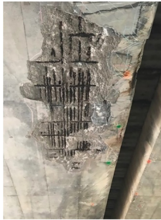
● Figure 2 Loose concrete removed
