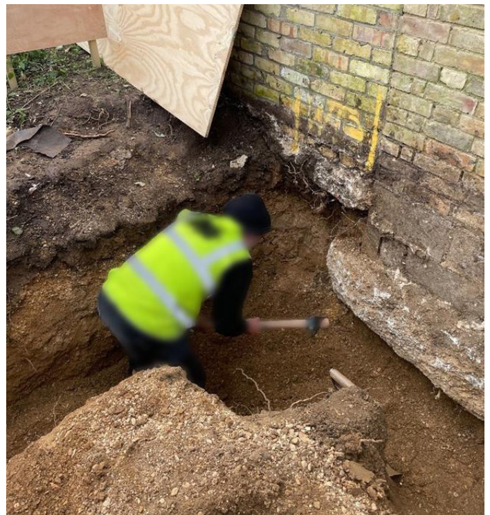
Figure 1: Unsafe excavation undermines masonry wall
