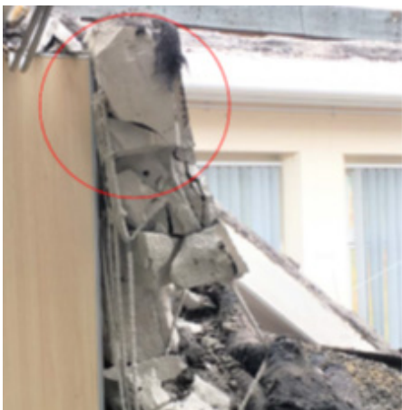
Figure 1: RAAC roof collapse at a school in 2018
