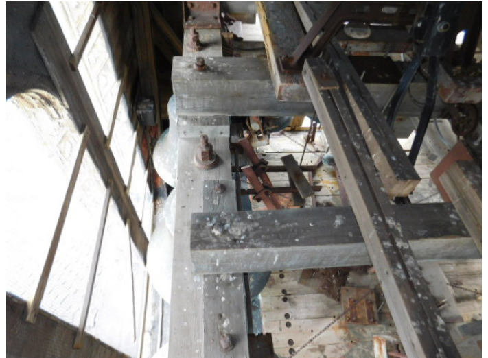
Figure 1: Timber structure supporting bells is structurally isolated from the exterior masonry walls
