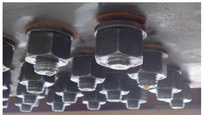
Figure 2: a loose tension control bolt after completion of joint
