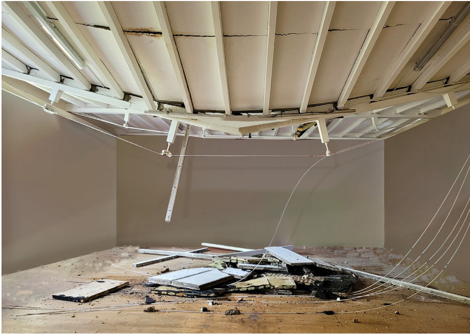
Figure 1: failed truss and partially collapsed roof
