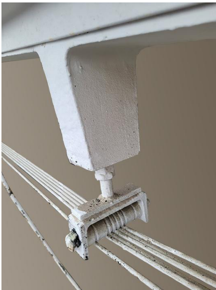
Figure 4: steel mount on concrete vertical carrying tensioned strands
