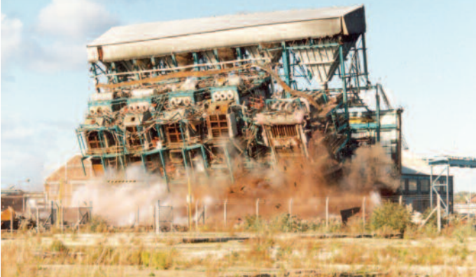
Demolition of the five coal-fired boilers on former chemical manufacturing site at Widnes. Copyright J Wolstenholme ©
