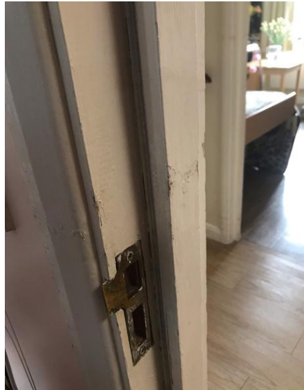
Fire door rebate showing intumescent strip fitted incorrectly
