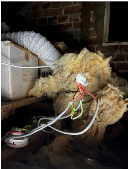
Faulty electrical installation that caused overheating and a fire alarm activation
