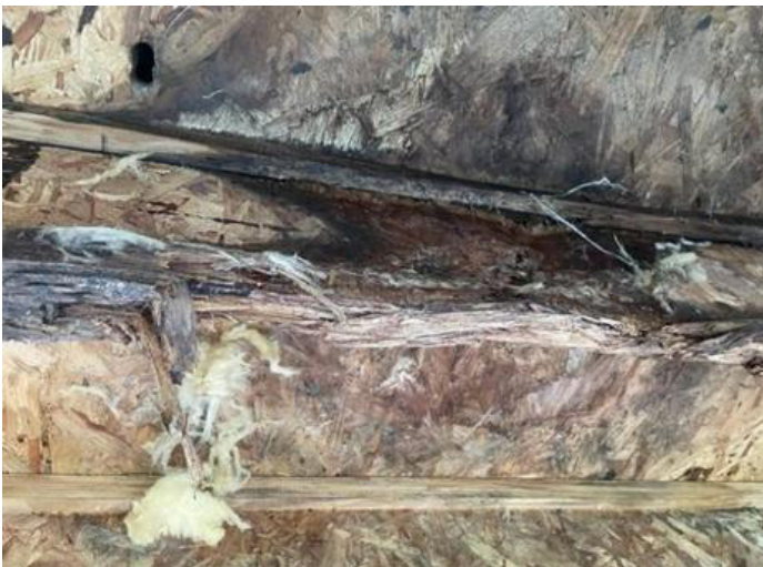
Figure 1: An example of OSB board deterioration
