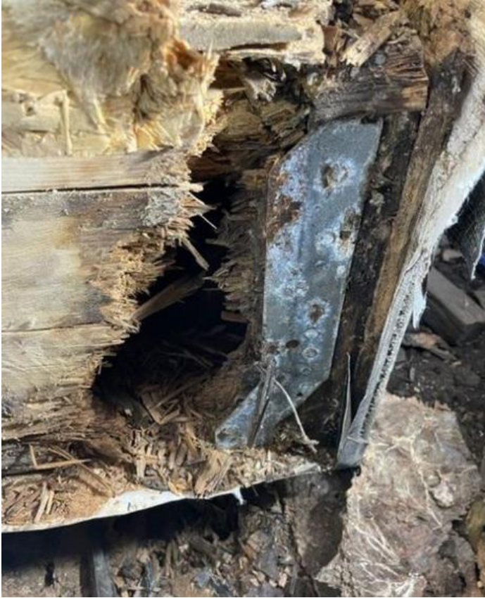
Figure 3: Engineered timber joist deterioration
